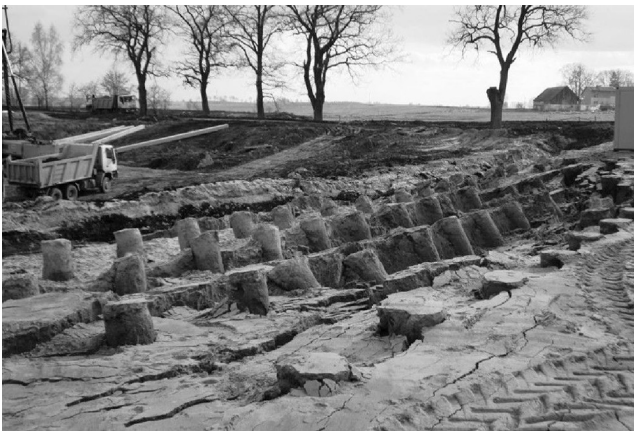
Figure 5.3 Damage to vibro concrete column heads caused by uncontrolled heavy site traffic. (Courtesy of Keller Group plc, London, UK.)
