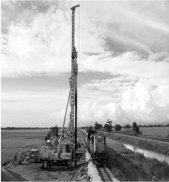
Figure 4.38 Vibrocat in operation next to existing railway track. (Courtesy of Keller Group plc, London, UK.)
