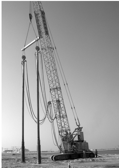
Figure 3.41 Vibro compaction equipment set up for S700 twin vibrator operation. (Courtesy of Keller Group plc, London, UK.)
