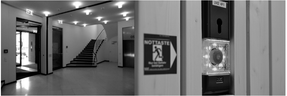
Fig. 43: Examples of emergency and security illumination
