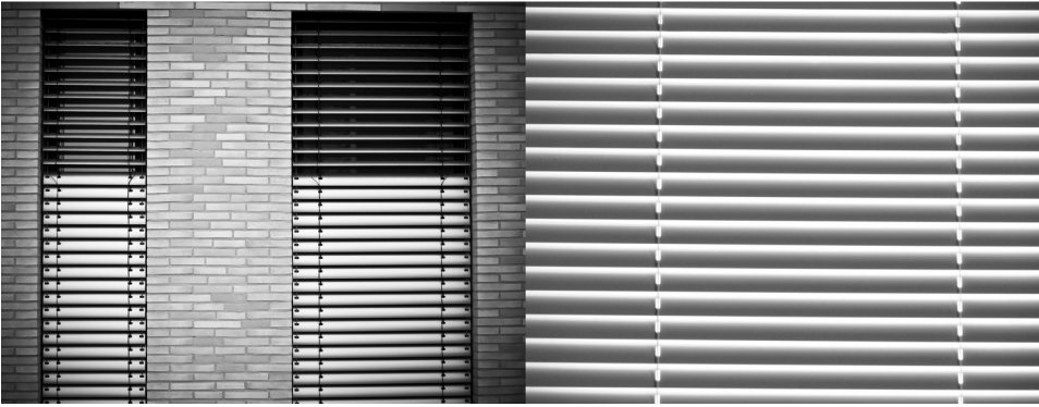
Fig. 11: External venetian blinds in laminated metal
