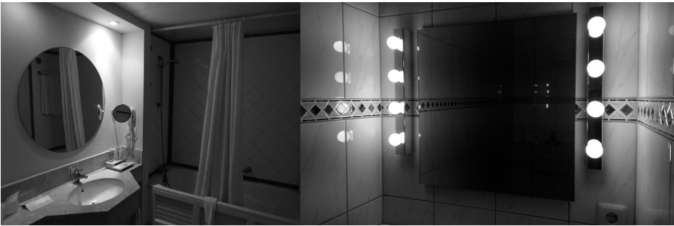
Fig. 48: Bathroom illumination and mirror luminaires
