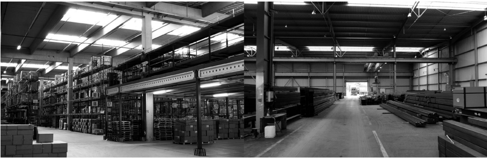
Fig. 42: Examples of warehouse lighting
