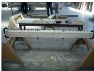
Fig. 6.13: Laminated beam built by insertion of long dowels through 4 wood layers using a sunflower oil welding retardation system.
