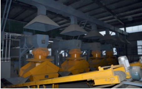
Fig. 5.41: Briquetting equipment and dust collector.
