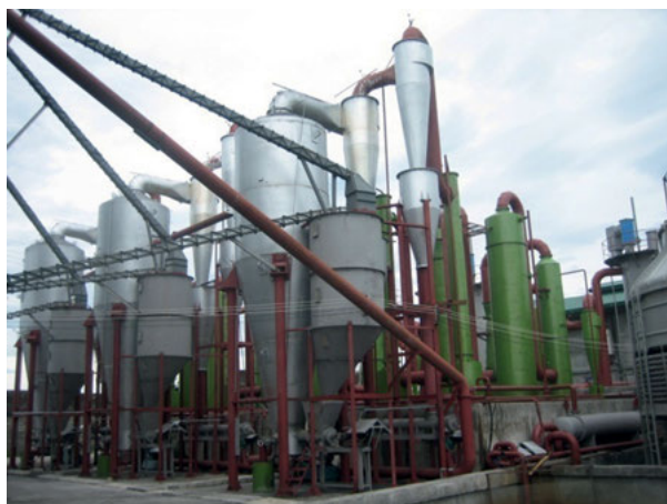
Fig. 6.22: Site view of the Philippine biomass gasification power generation project.
