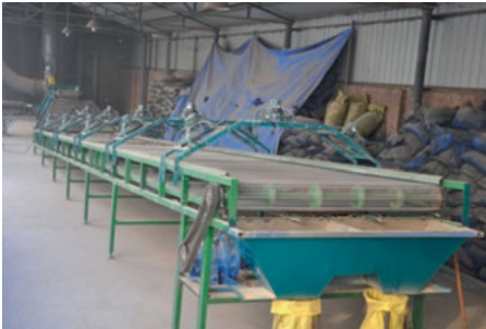
Fig. 5.49: Cooling and drying system.
