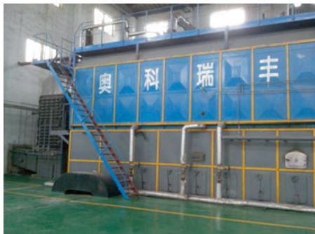
Fig. 5.51: Biomass boiler of the Excelic Food Technology Company.
