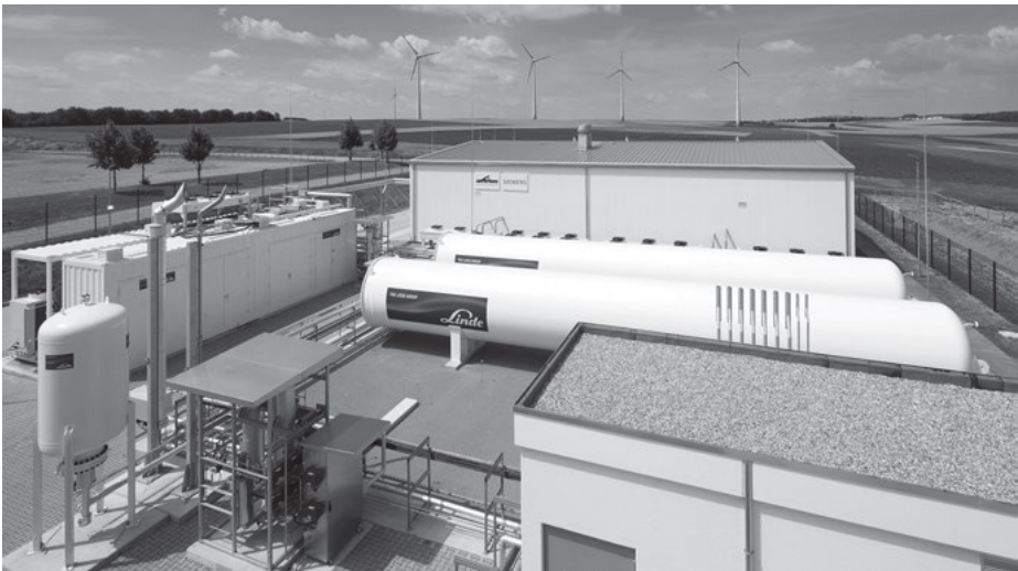
Figure 7.20: Power-to-gas installation of the Energiepark in Mainz (Energiepark Mainz).
