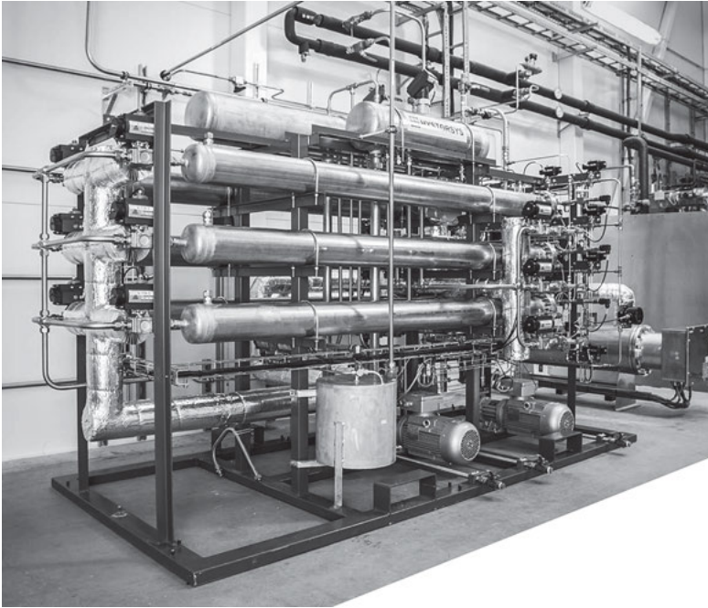
Figure 5.8: Two-stage thermal compressor (Hystorsys AS).
