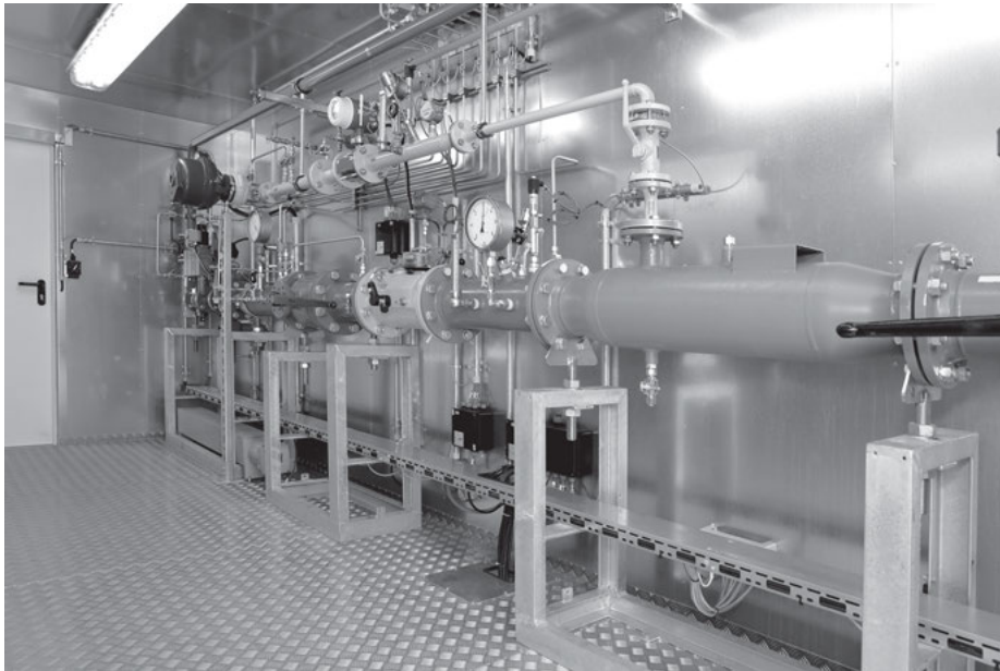
Figure 7.12: Hydrogen injection station in the natural gas network (Thüga / Mainova).
