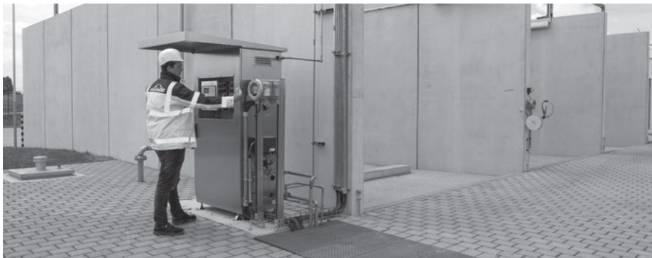
Figure 7.23: Hydrogen service station (Energiepark Mainz).
