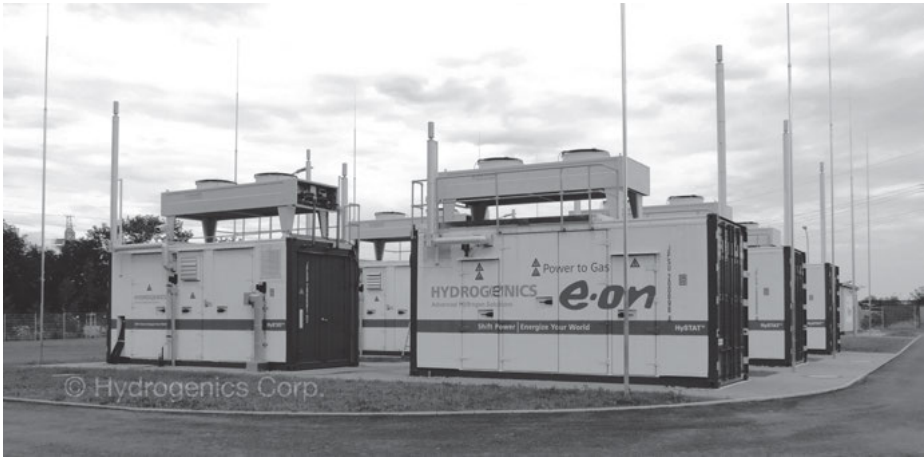
Figure 7.30: Electrolysers of the Falkenhagen power-to-gas unit (Hydrogenics Corp.).
