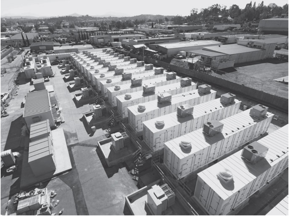
Figure 2.15: Storage park with capacity of 30 MW (San Diego Gas and Electricity).
