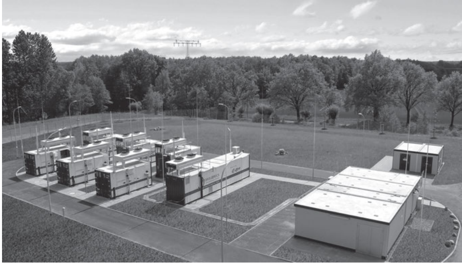
Figure 7.28: Falkenhagen power-to-gas unit (E.ON).
