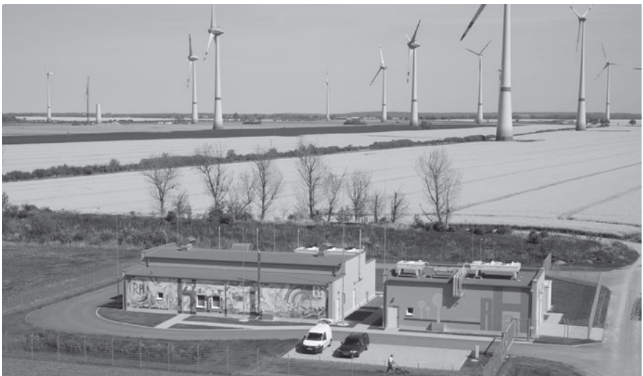
Figure 7.17: RH2-WKA installation (WIND projekt GmbH).
