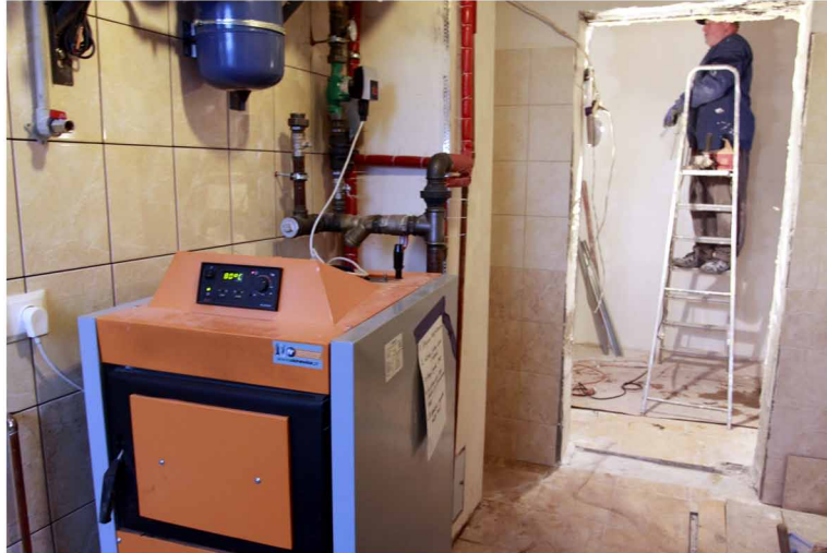
Figure 7. New heating and domestic hot water installation; The new wood gasification boiler is visible. KAPE SA, 2016.
