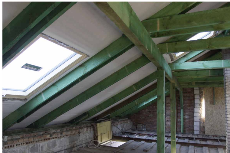
Figure 5. Attic after reinforcement of rafter framework and ceiling; Roof windows already installed KAPE SA, 2016.
