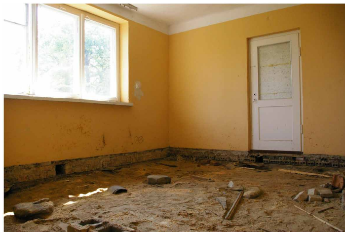
Figure 2. Taking apart the floor: The stones visible were used as support for floor joists, wall vents are also visible. KAPE SA, 2016.
