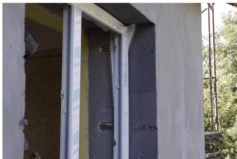
Figure 6. Window installation in the wall's thermal insulation layer on steel consoles KAPE SA, 2016.
