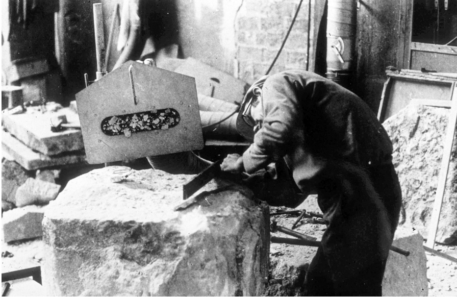
Figure 2.2 Honest toil – master stonemason at work on site. Contrast this with the situation in Figure 2.12, where all stone-cutting is undertaken off site.
