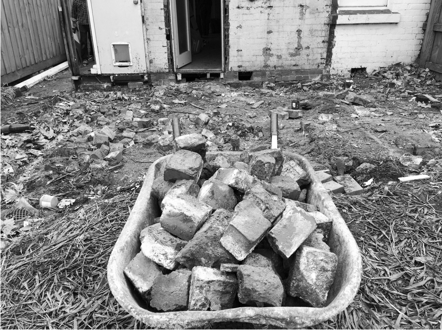
Figure 5.4 After the timber kitchen and bathroom had been removed the underfloor area was full of broken bricks of the same red clay as the old house structure.
