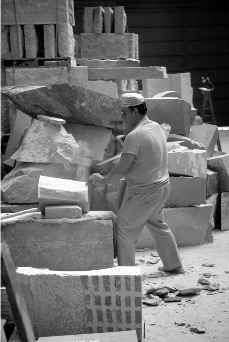
Figure 2.1 Until 1989 nearly all the stone was dressed on site using saws where possible, and manual techniques to complete the task: highly skilled work, tough on the muscles as well as the ears and lungs.
