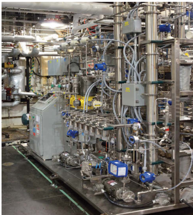
Figure 2.2: The demonstration unit for wastewater purification, built by Forward Water Technologies in Mississauga, Canada.
