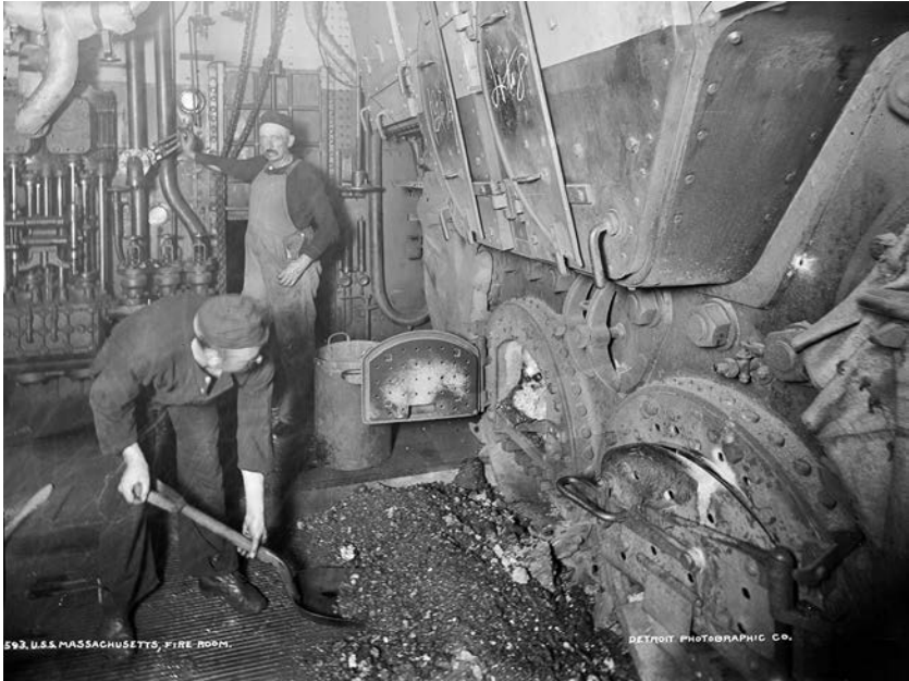
Down in the boiler room. The USS Massachusetts fire room, late nineteenth century. Edward Hart/Library of Congress
