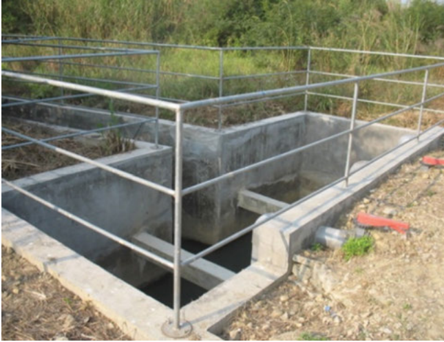
Figure 6.5: Lift pump station.
