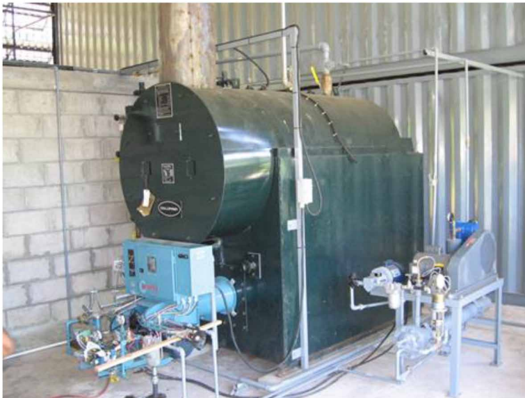
Figure 5. Showing boiler equipment and boiler using waste motor oil as number 2 fuel to produce steam for cooker
