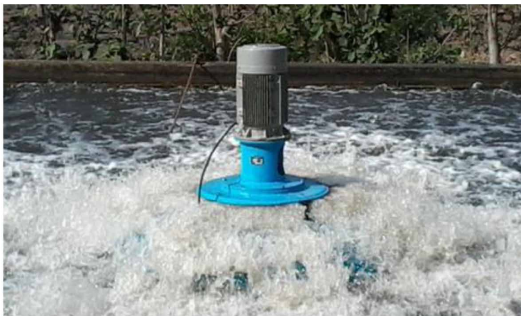
Figure 7. Mechanical aerators with blades or brushes
