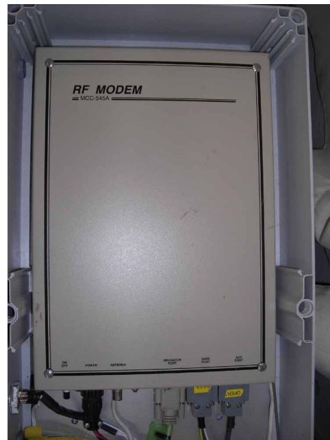
Figure 2d. Lake Saroma remote station: Transceiver (called RF MODEM) MCC-545A manufactured by MCC, installed in a duralumin box
