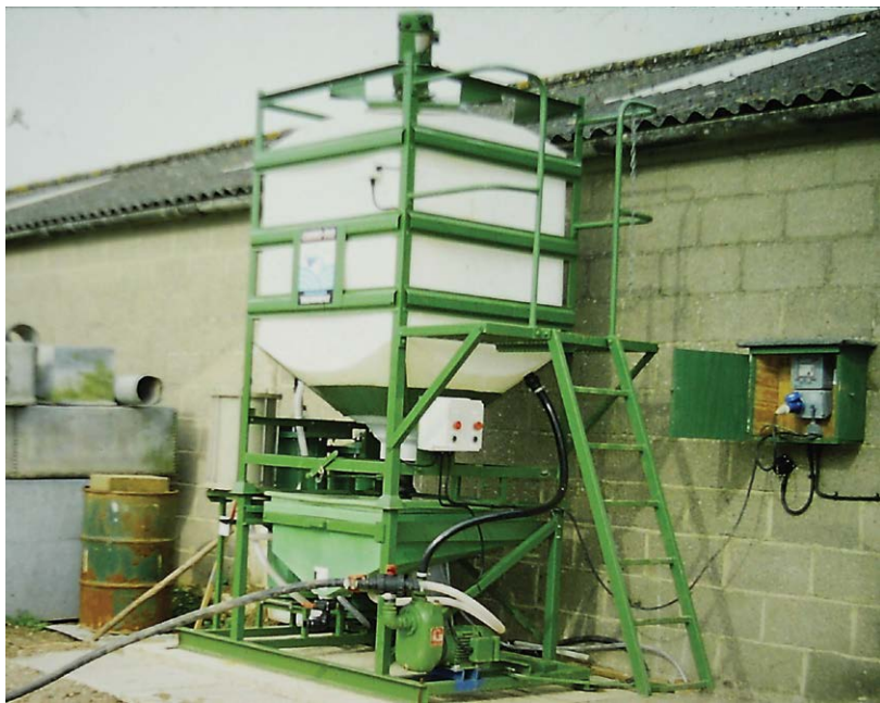
Fig. 9.22. A water treatment plant to remove pesticides from water used by sprayers operated by a contractor. (Photo courtesy of Sentinel, used with permission.)
