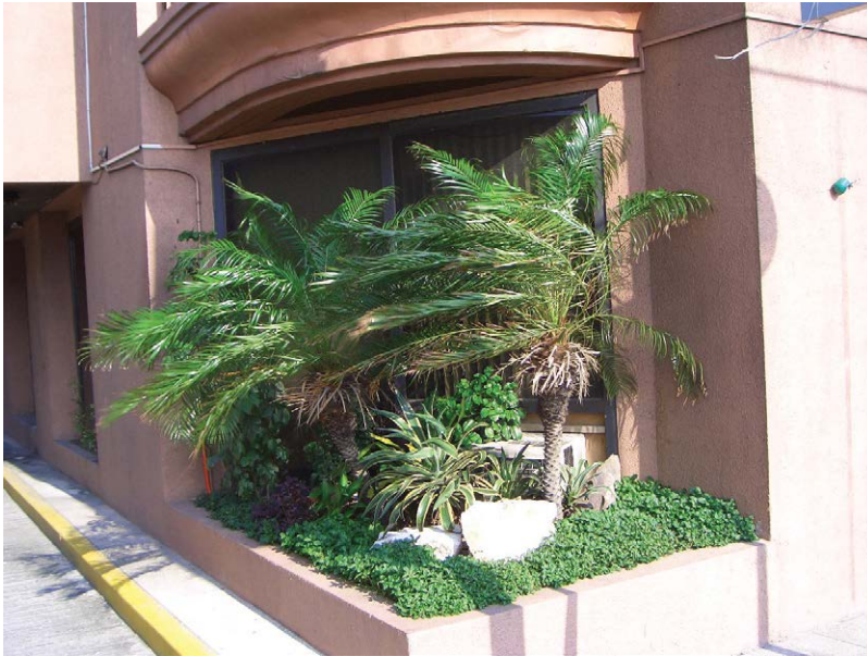
Fig. 6.22. Landscape and planter boxes in close proximity to a structure are significant reasons for termite infestations. (Author's photo.)
