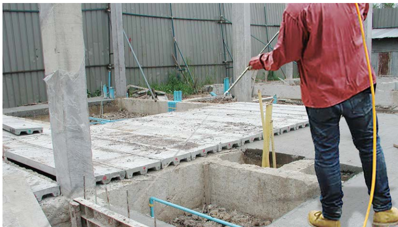
Fig. 6.30. Treating the soil at the foundation level before the start of construction. (Courtesy of Richard Tang.)
