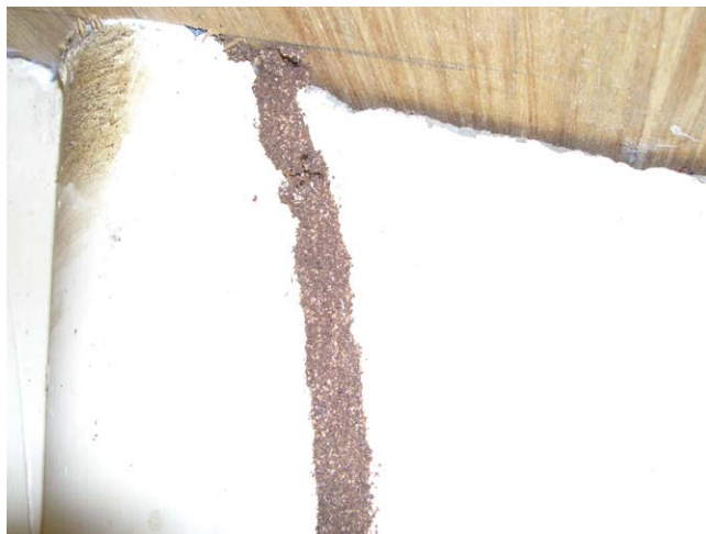
Fig. 6.17. Mud tube used by Nasutitermes sp. to access wood in the structure. (Author's photo.)
