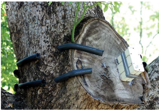
Fig. 11.16. (b) An above-ground station installed on an outdoor infested site. (Courtesy of Paul Yuen.)
