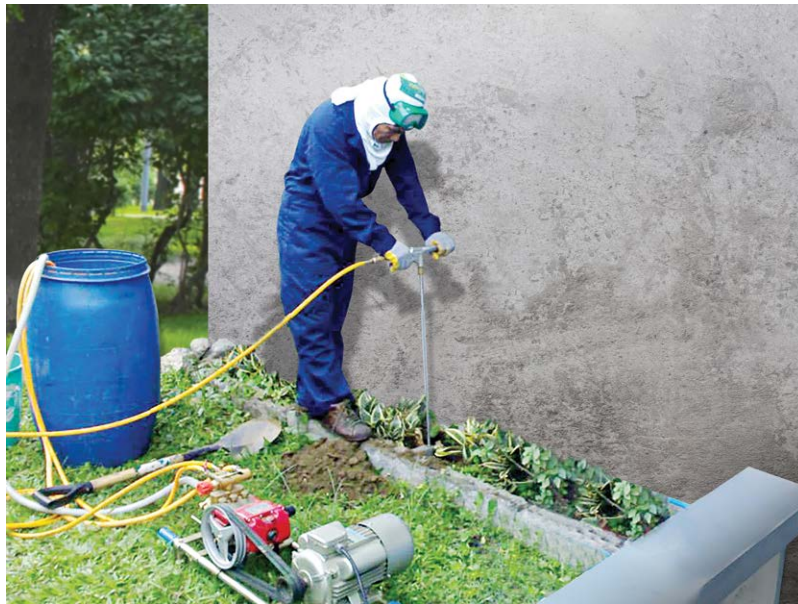
Fig. 6.26. Treating the soil outside the structure using a power machine. (Courtesy of Andrew Gok.)
