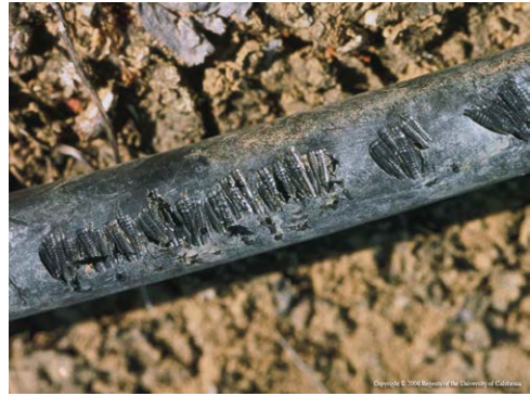
Fig. 16.15. Gnawing damage to drip irrigation pipe. (Photo by J.K. Clark, Copyright the Regents, University of California.)
