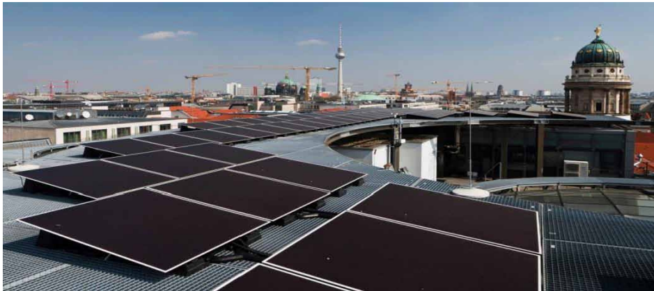
Figure 15. Solar panels on the roof of the Galeries Lafayette shopping center in Berlin
