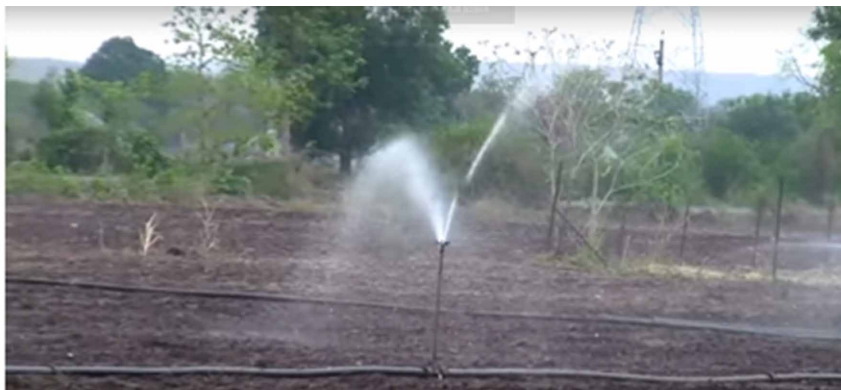
Figure 21. Semi- Permanent sprinkler irrigation system
