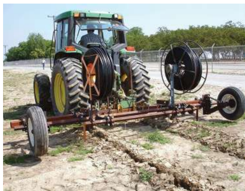
Fig. 10.1. Installation of subsurface drip irrigation tubing prior to planting a pomegranate orchard in California (USA). (Photo: Claude J. Phene et al. , 2015, University of California Agriculture and Natural Resources.)
