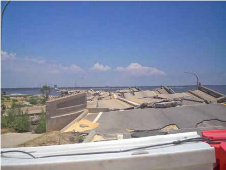
Figure 3.3 Destroyed Biloxi-Ocean Springs Bridge. Source: Created by Jennifer Trivedi.
