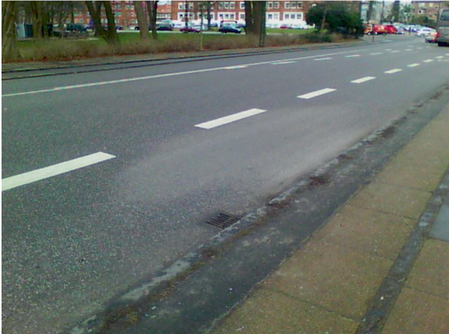
Figure 3: The site of the suspected leak. I would like to thank Søren Ernst (HOFOR A/S) for allowing me to use this photo.
