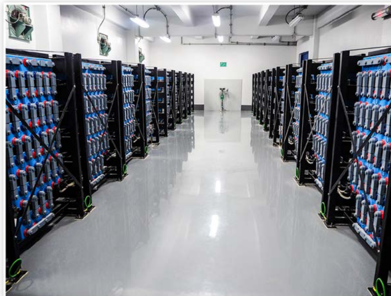
FIGURE 9.7 Battery room in power plant.
