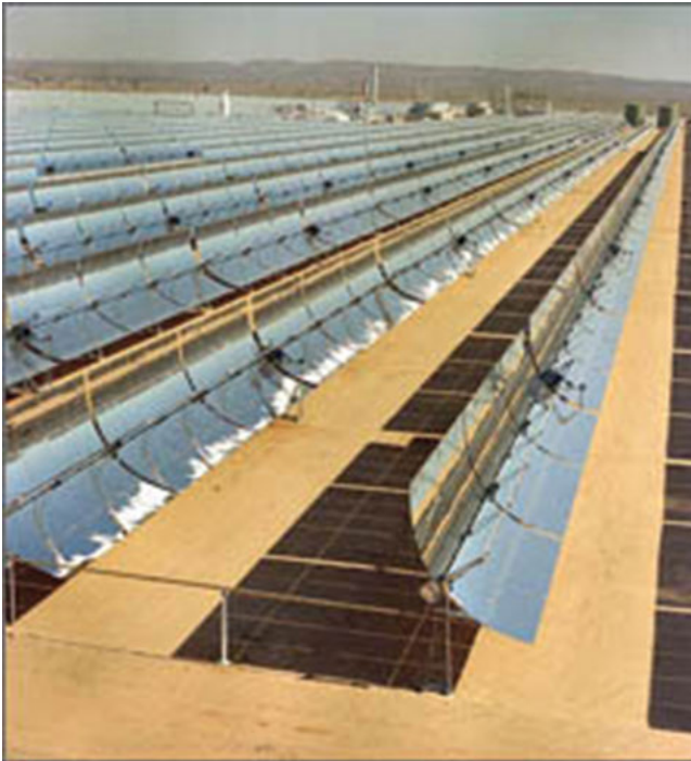
Figure 8.3: Parabolic troughs for CSP. (Photo, public domain, courtesy of National Renewable Energy Laboratory)
