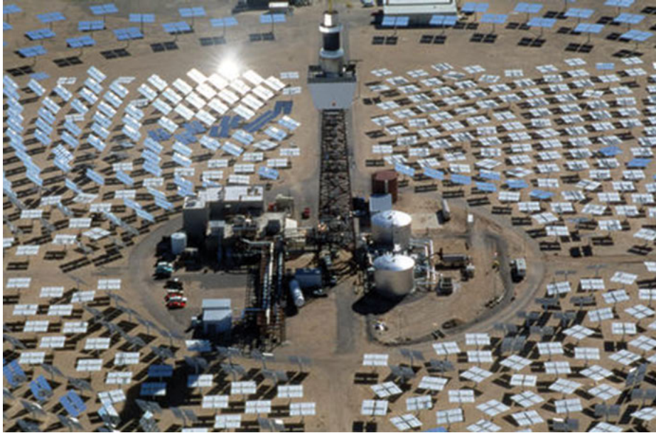
Figure 8.4: Solar power tower CSP. (Photo, public domain, courtesy of the National Renewable Energy Laboratory)
