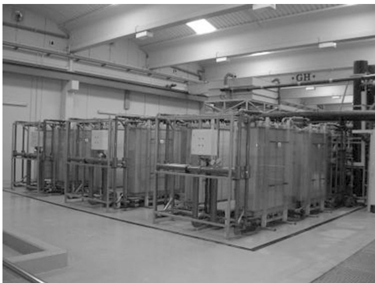
Fig. 12.1: EDR technology of the company MEGA a.s. for production of irrigation water from municipal wastewater after biological treatment in the Depurbaix area (Spain) (photo: MEGA a.s.).
