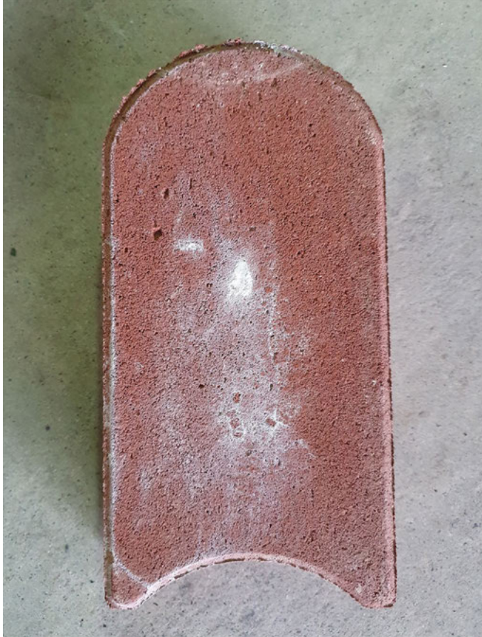
Figure 16.4: Paving slab showing the effect of efflorescence.
