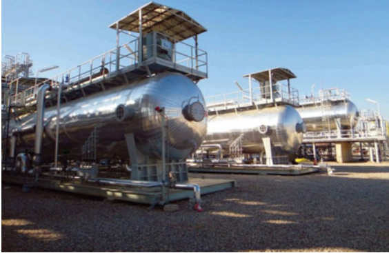
Figure 4.14: Crude oil desalting unit. From https://howebaker.com/wp-content/uploads/2017/07/Desalter-1-768x495.jpg .
