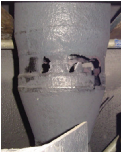
Figure 6.27: FCC cyclone damage by erosion.
