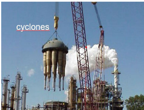
Figure 3.4: Cyclones for a fluid catalytic cracking reactor.
