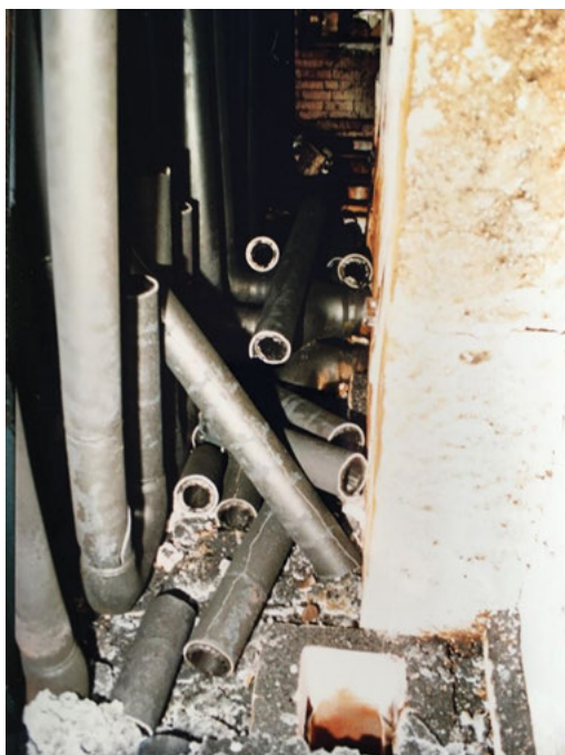
Figure 6.38: Collapse of the furnace coils (from https://media-exp1.licdn.com/dms/image/C5122AQE7sciD9B54-Q/feedshare-shrink_2048_1536/0/1577899217620?e=1623888000&v=beta&t=KmdrM_cx_Em3NjRlflcXr3xQlUWZNTj-W2u0sfDvjDI ).
