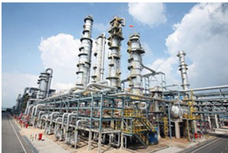
Figure 9.40: The propane-based plant of Asahi-Kasei for manufacturing of acrylonitrile ( https://www.asahi-kasei.co.jp/asahi/en/news/2012/images/e130213_1_02.jpg ).
