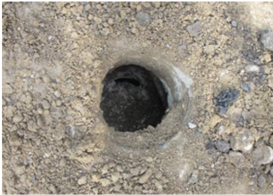
Figure 1-3 Photograph of the damage to the medium pressure DN500 gas line
