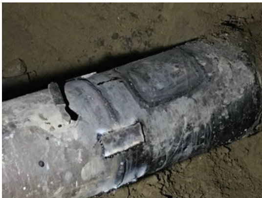
Figure 1-6 Gas pipeline weld defects.
