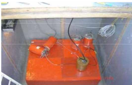
Figure 6. Geotech and Reftek digital broadband seismic sensors housed inside the vault
