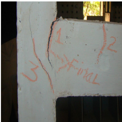
Fig. 5. Cracks in S3 Specimen
