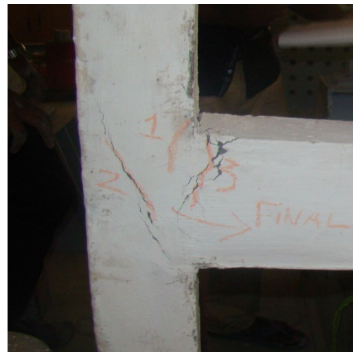
Fig. 6. Cracks in P1S3 Specimen
