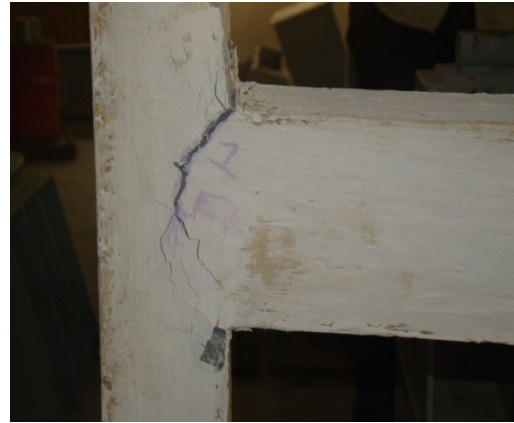
Fig. 4. Cracks in P1 Specimen
