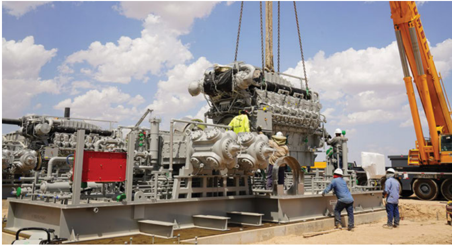
Figure 10.4: Safe lift of a major gas engine onto its base (courtesy of CES L.P., www.ceslp.net ).
