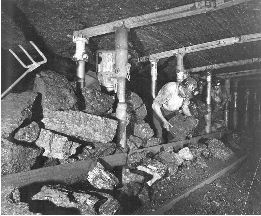
Figure 4.7 Miner hand-loading large pieces of coal onto a face conveyor (photo credit: Coal Authority)
