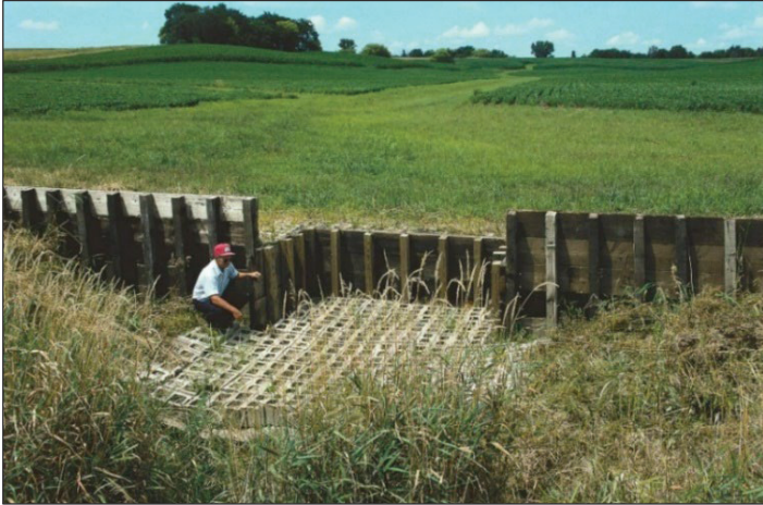
Figure 5.10 A drop structure made of timbers and concrete blocks stabilises a grassed waterway channel in Iowa, U.S. The waterway extends hundreds of metres up through the surrounding crop fields, safely conveying runoff water away, while the structure prevents a gully from forming in the channel (Photo credit: USDA-NRCS).
