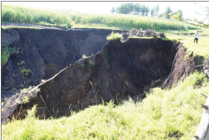
Figure 5.4 Classical gully in northeast China. The eroded channel has destroyed a road and is encroaching into adjacent fields (Photo credit: USDA-ARS).
