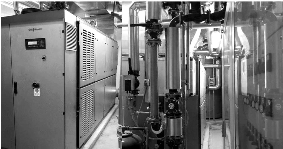
Figure 9. Nonpolluting energy that powers factory one (source: Cubo Design official website)
