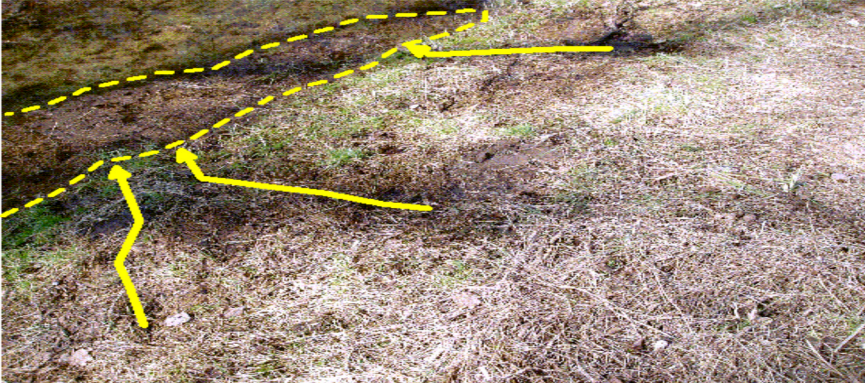
Figure 3: Detail of seepage at the levee base under flood conditions.
